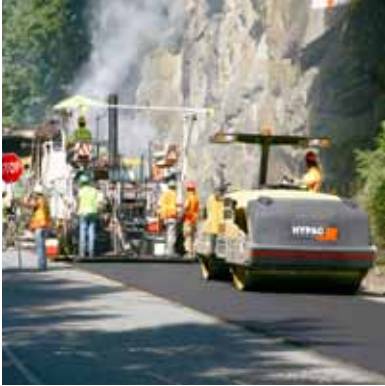
Road resurfacing is a scheduled maintenance task required to keep a high quality transportation system.
